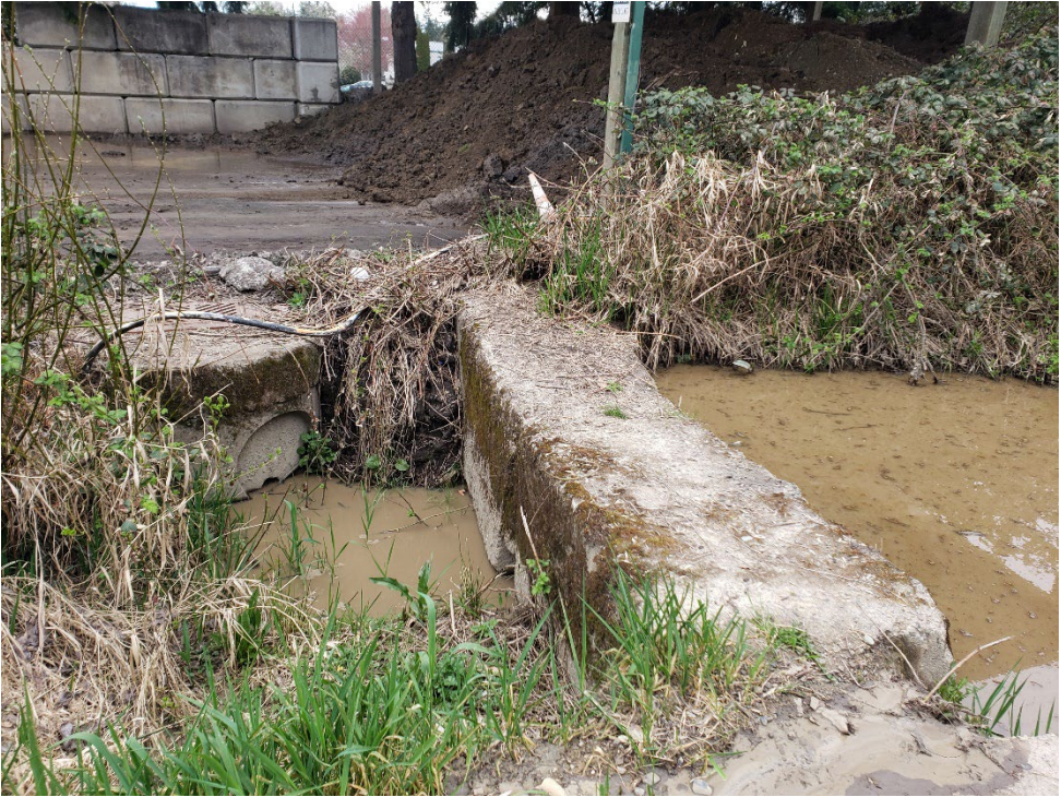
Photo 24. Type 2 catch basin (2a-82), adjacent to stormwater feature.
