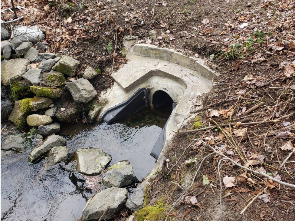
Photo 14. Piped section of Stream A along private access road to Public Works facility.
